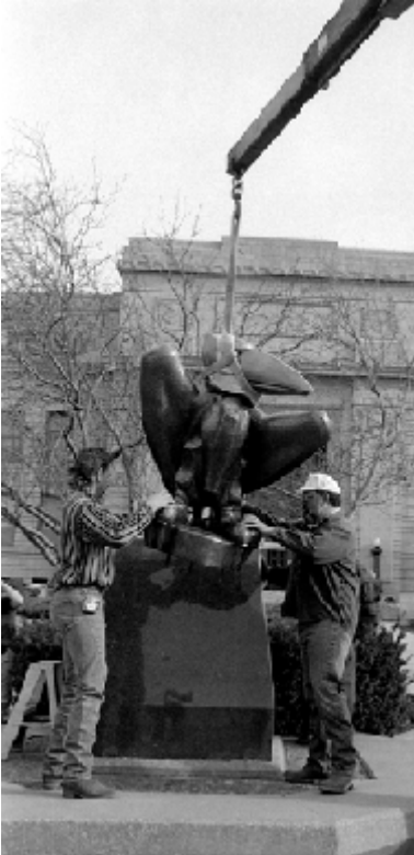
"Jayhawk" by sculptor, Elden Tefft of Lawrence, KS, being reset on its base following repairs and refurbishment.
